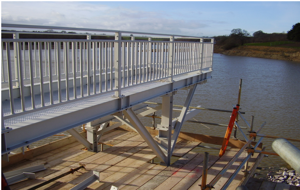
Figure 3 - New bridge providing access to valve spindles and actuators
