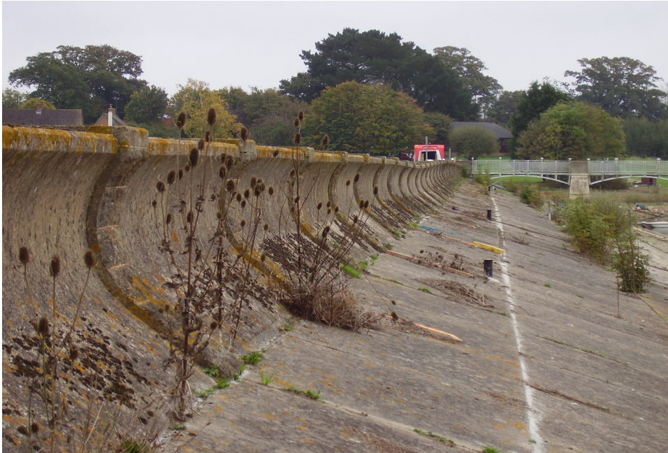
Figure 4 - Wave wall and concrete slabbing prior to the start of the works
